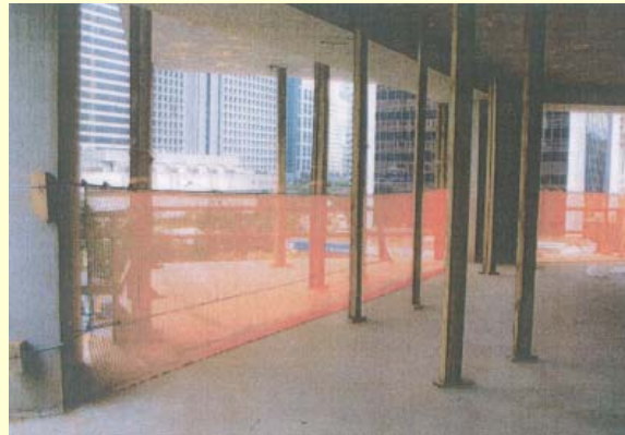
d) Finally, on each new floor under construction, a dense fence, as shown above, will be erected inside the perimeter of the building edge (also employed in Phase 1).
