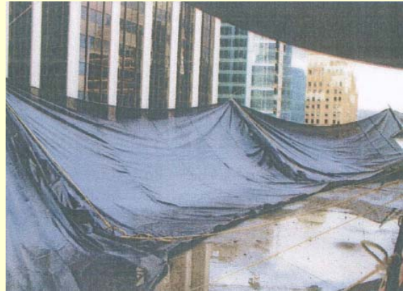
c) Below each newly constructed floor (and moving up as construction proceeds) will be a 20-foot wide resilient net extending outward from the building. This measure (shown above) was tested and employed in Phase I construction.
